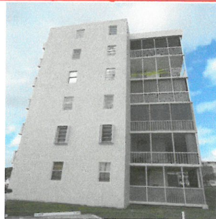
No Opening Protection
